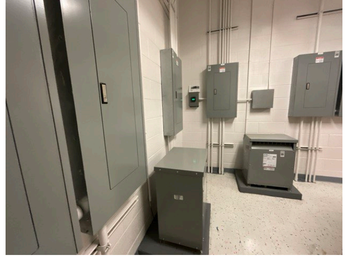
20 - MAIN ELECTRICAL ROOM
