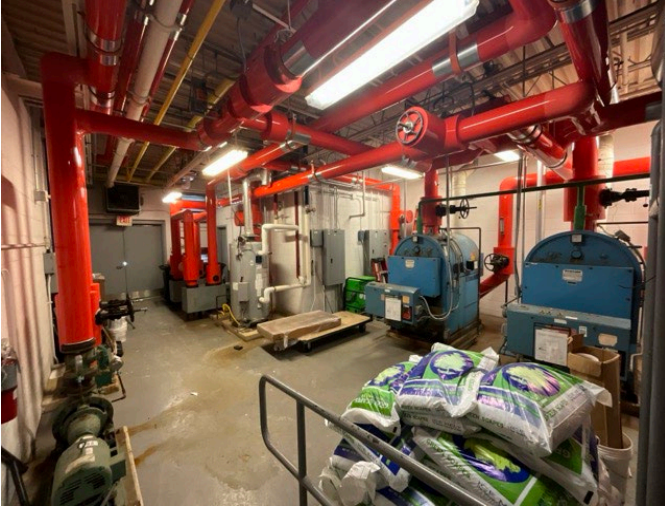
19 - MAIN MECHANICAL ROOM
